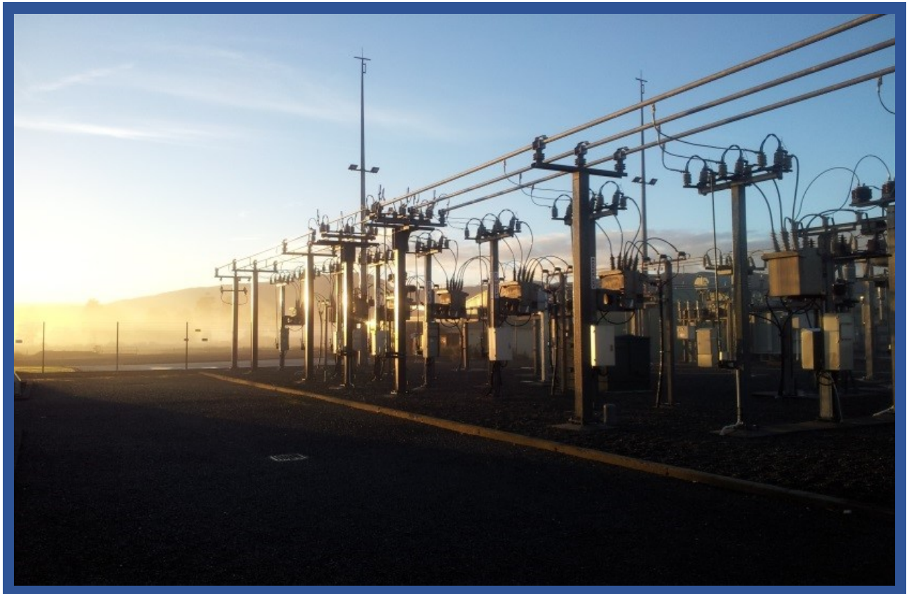
Robertson Substation Westport
