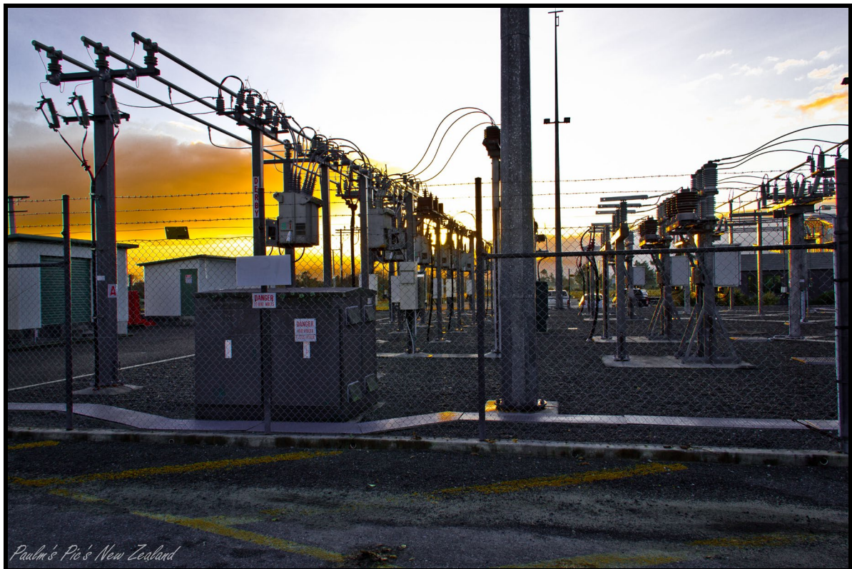
BEL Robertson Street Substation Sunrise
